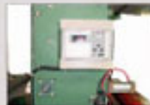
ELECTRIC TENSION CONTROL
