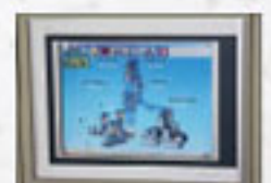
HMI CONTROL (TOUCH SCREEN)
